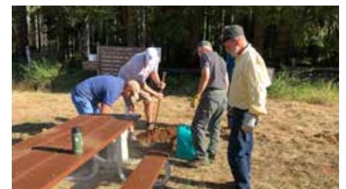
Above: Enjoying McKenzie Bridge State Airport; Below: Anchoring the new picnic table at July work party
